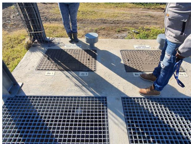
Circulation and Reticulation Pumps
