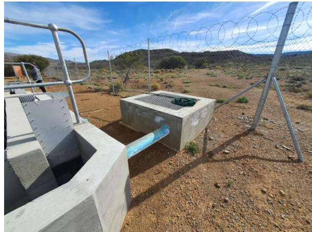
WWTW (Inlet Works)
