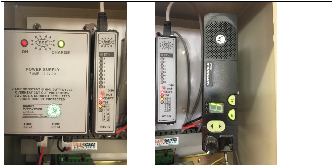
Power Supply and Motorola CM140 radio at the Control Station.
