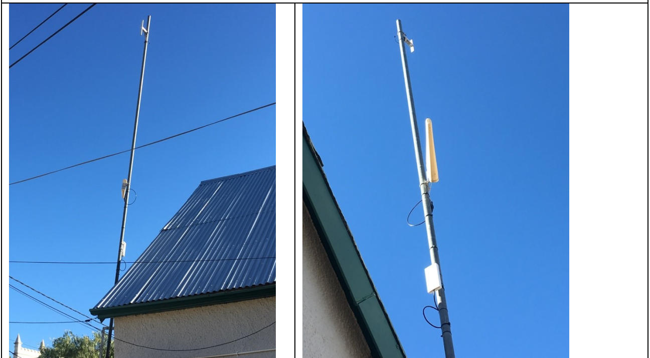
Existing Telemetry Antenna at the Control Station.
